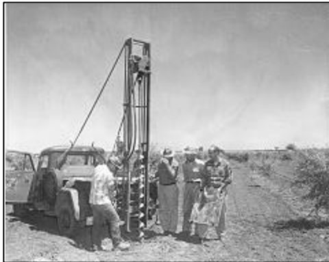
Water table level investigations are being made by the directors and SCS engineers preliminary to the development of specifications for placing of tile drains. Cooperators have installed about 3 miles of tile drains in 1959.
